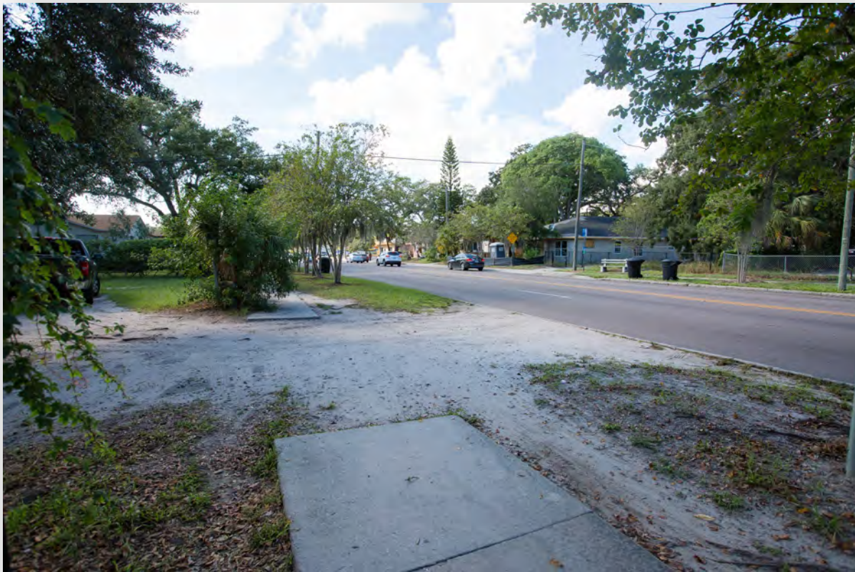
Interrupted sidewalk on 18th Avenue South
