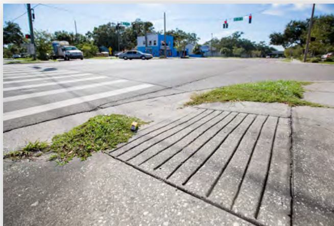
Overgrowth on a curb ramp
