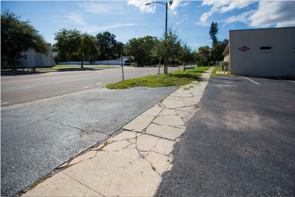
Cracked sidewalk along 18th Avenue South
